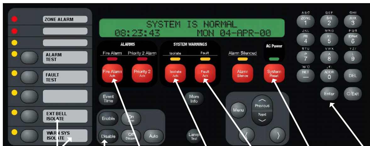
OUTPUT ISOLATES DISABLE FIRE ALARM ACK ISOLATE ACK FAULT ACK SYSTEM RESET ENTER
